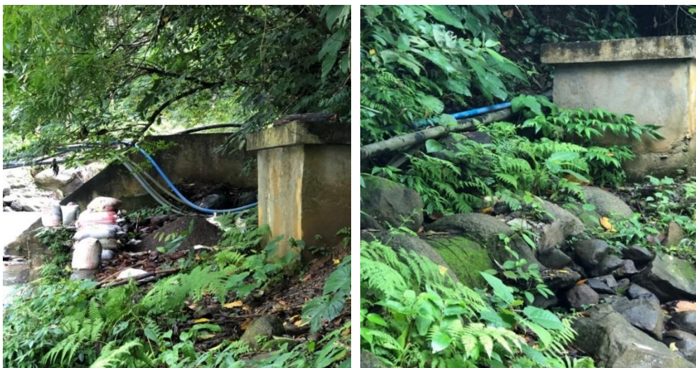
Some of the structures of the main diversion works, including a partly damaged reinforced concrete pipe
