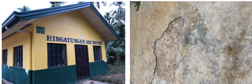
The Hingatungan Post-Harvest Facility building and a portion of the sun-drying concrete pavement with detached surface plastering
