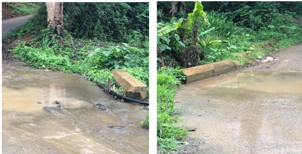
Waterlogged and damaged portion of the Pitogohan-Iyusan FMR near an existing culvert
