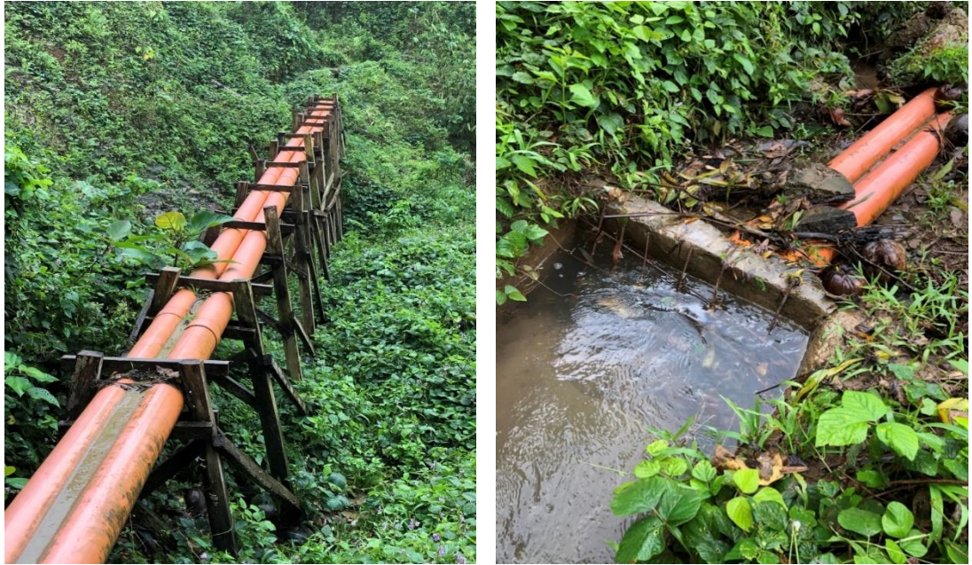
The temporary (PVC-pipe) flume that replaced a portion of the original one destroyed during the landslide, clearly showing the reduction in the discharge volume
