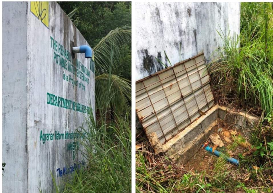
The reservoir of the Hingatungan Potable Water System showing two sizes of outlet pipes
