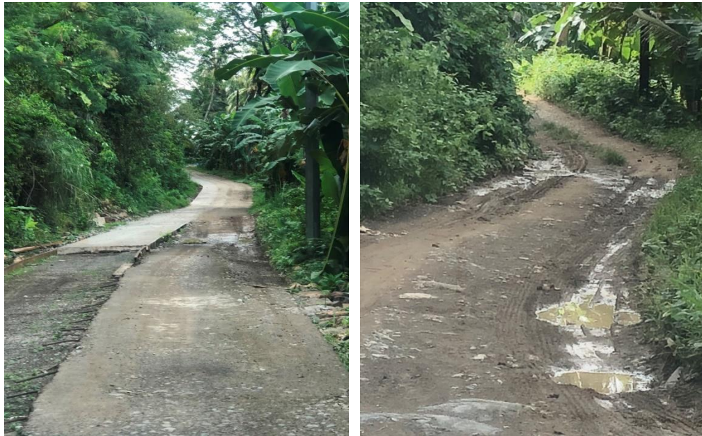
The Pinut-an-Kinachawa FMR showing water-logged portions, collapsed pavement and poorly constructed portions that exposed the coarse aggregates
