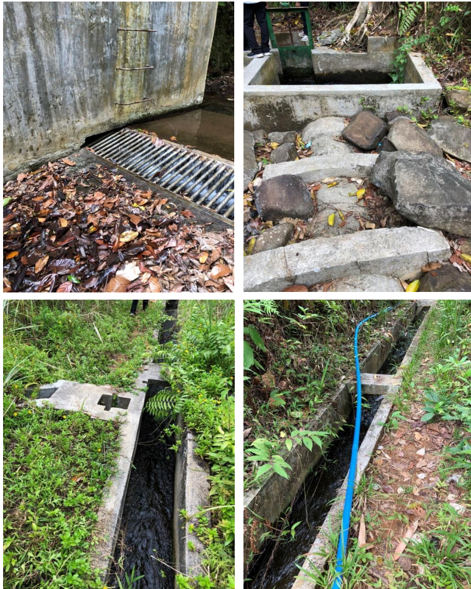
The Katipunan Irrigation Project
