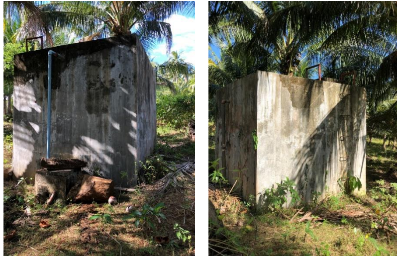
The Balaquid potable water system reservoir
