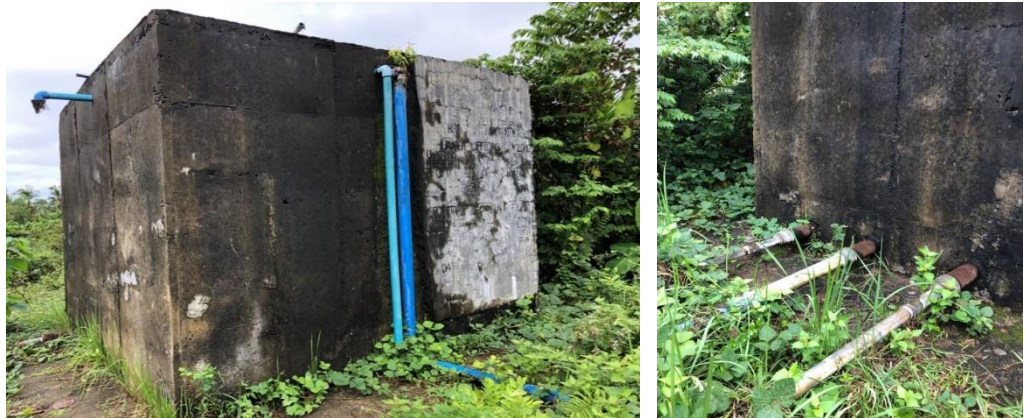
The reservoir showing the intake pipe (left) and the three (3) outlet pipes (right) after the ARISP III project
